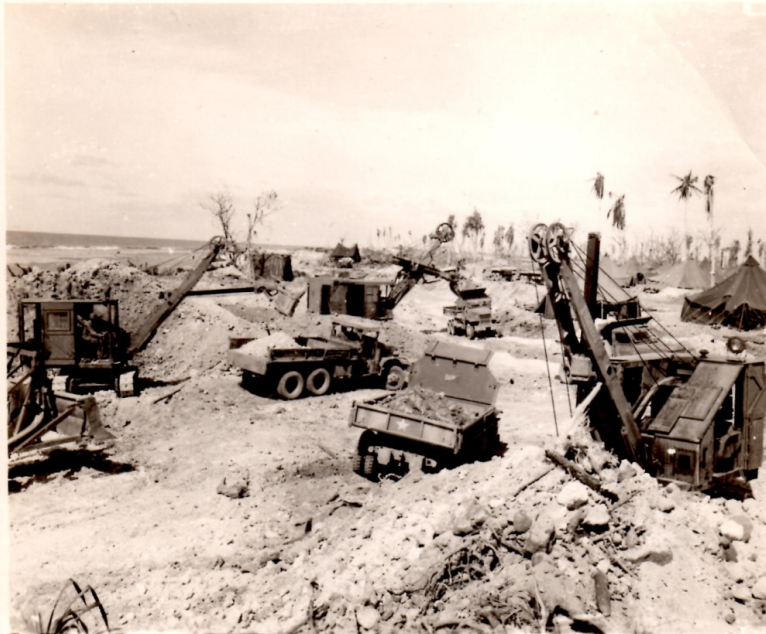
КШАЖАЛЕИМ 20 FEBRUARY 1944 POWER SHOVELS DIGGING SUBGRADE MATERIAL NEAR THE OUTER EDGE OF THE ISLAND.
