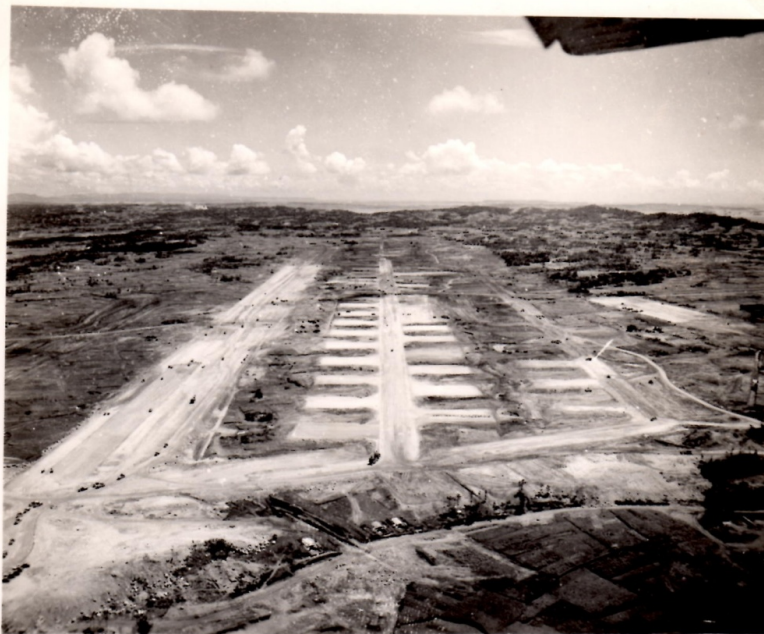
OKINAWA 12 AUGUST 1945 JUST BEFORE JAPAN'S SURRENDER OFFER WAS ACCEPTED FUTEMA AIRFIELD CONSTRUCTION HAD REACHED THIS STAGE.
