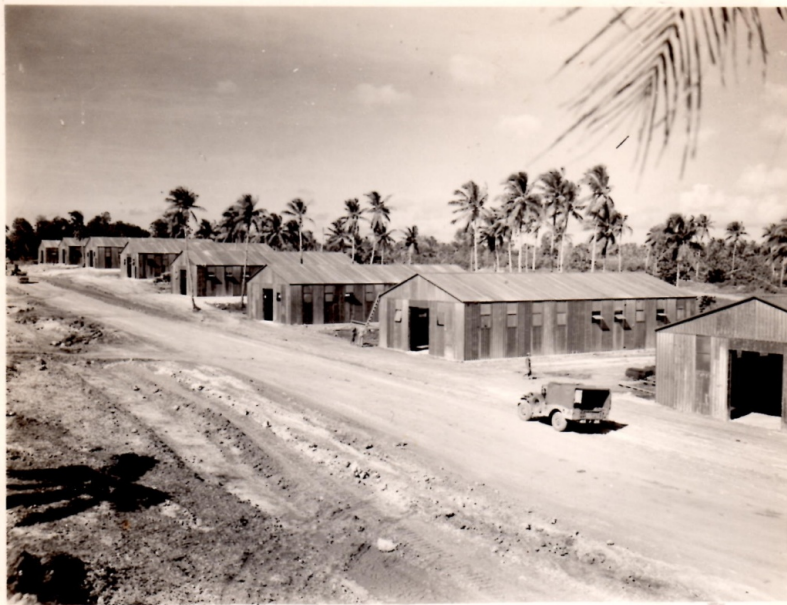
GUAM 24 NOVEMBER 1944 COMPANY B AVERAGED ERECTION OF ONE STRUCTURE EVERY TWO DAYS IN CONSTRUCTION OF BUTLER STEEL WAREHOUSES.
