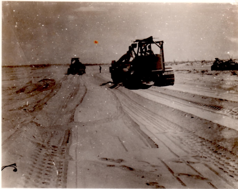
LAGUNA, ARIZONA 20 AUG. 1943 SWELTERING SUN AND DESERT SAND WERE EVERPRESENT DURING LAGUNA AIRFIELD CONSTRUCTION.
