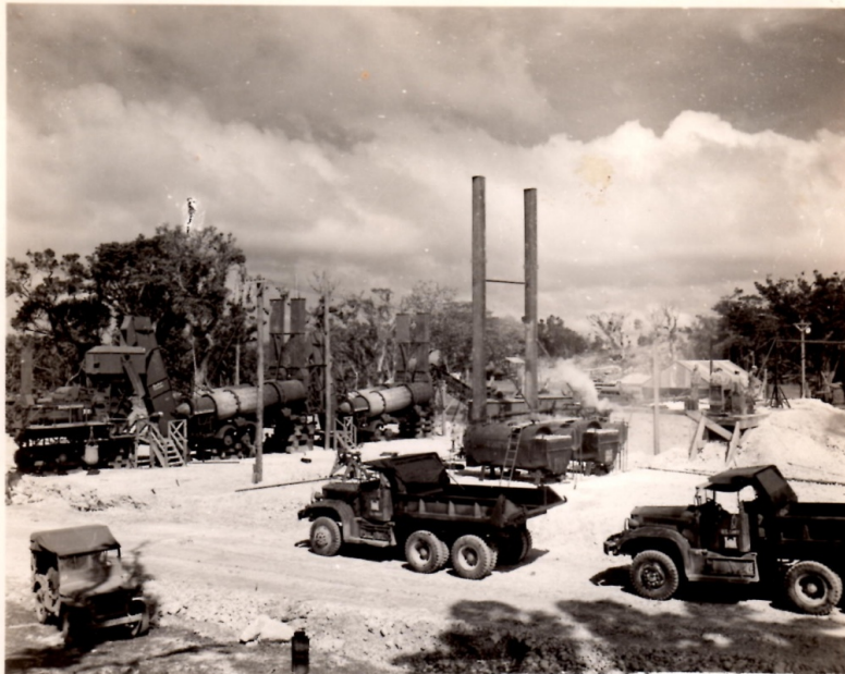
GUAM 16 JANUARY 1945 EVERYTHING IS IN READINESS TO START THE ASPHALT PLANT. SHOT WAS TAKEN DAY BEFORE OPERATION COMMENCED.
